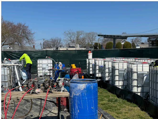
Permeable Reactive Barrier Injection Wells in Lake Agawam Park
